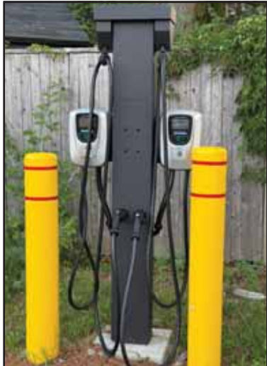
CHARGING STATIONS PERLEY SCHOOL Contract bids managed by Georgetown Elect. Light Dept. Selected Contractor: ACI TOTAL PROJECT COST: $36,264
