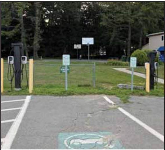
CHARGING STATIONS AMERICAN LEGION PARK No bids, managed by Town Admin. Orlando Pacheco. Contractor: Inovis TOTAL PROJECT COST: $59,226
