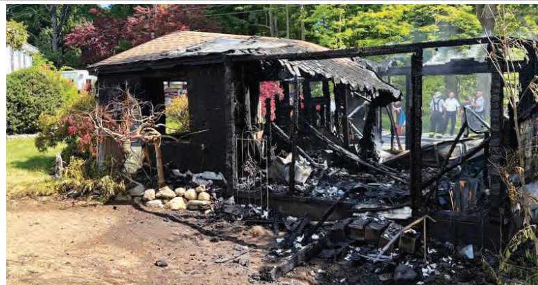
A detached garage at 79 Church St. in West Newbury (Photo courtesy West Newbury Fire Department)
