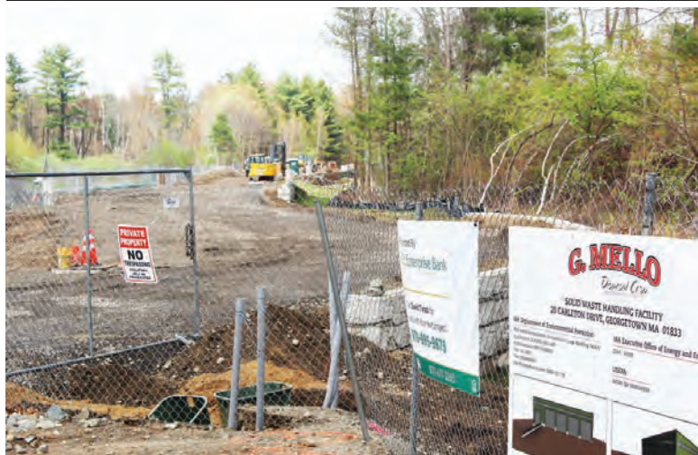
Mello's huge transfer station construction site: Earthworks makes way through wooded area adjacent to 195. (Photo: Stewart Lytle)
