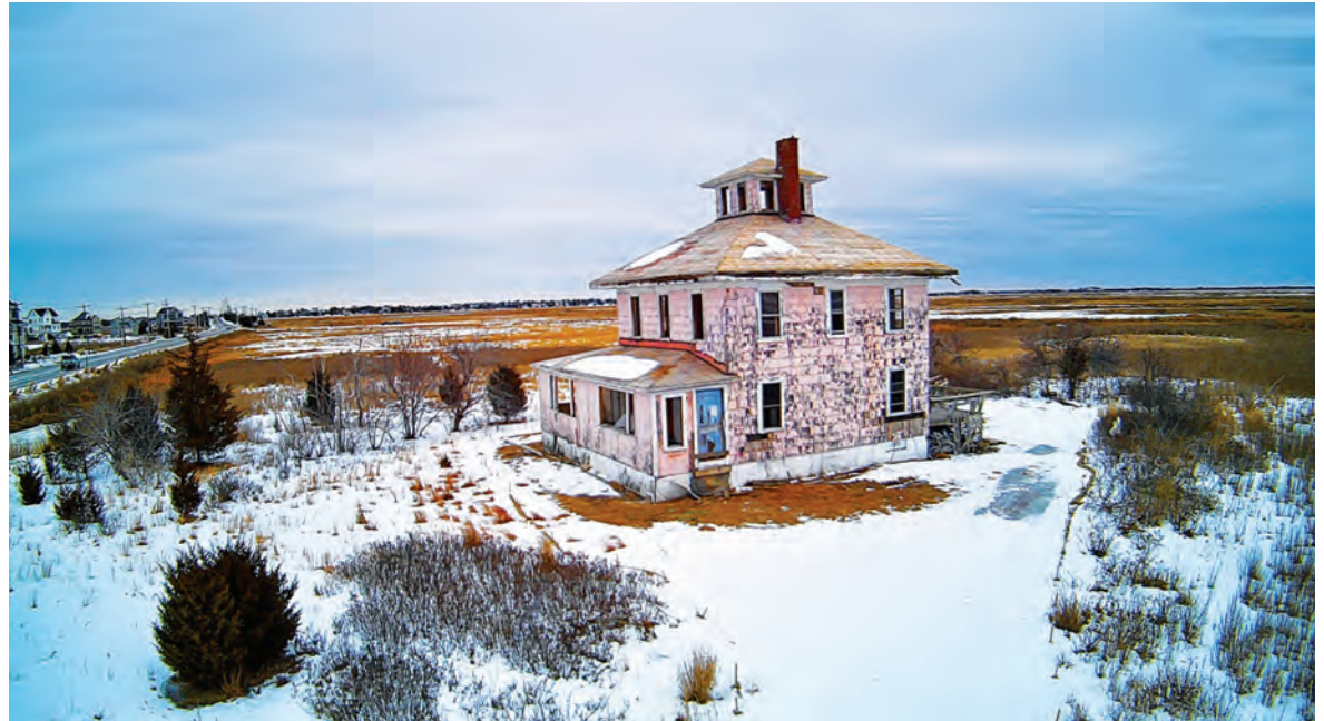
The iconic Pink House, stripped of its roofing and most windows and subjected to planned decay by the federal government for years, silently awaits demolition. (Photo: Lomie Brennan)
