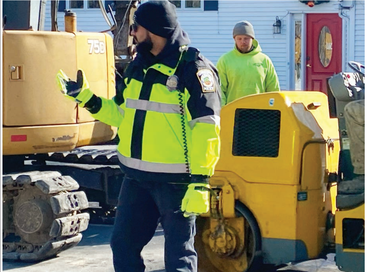
Georgetown Police Officer Tristan Straker directs traffic in frigid, single-digit weather while a crew from Joseph P. Carillo & Son, Inc. complete emergency winter repairs on a huge vehicle-hurling pothole and depression (apparently caused by a water issue). The final patch measured more than 8 x 4 feet on busy Rte. 133 / Andover Street last week. (Photo: Lonnie Brennan)
