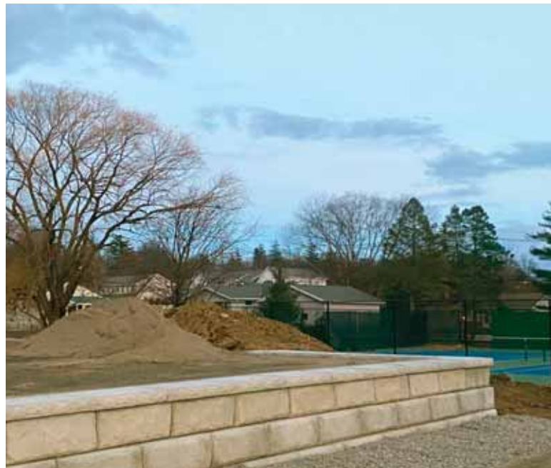
Photo taken last weekend shows section of new elevated retaining wall, gravel, and dirt piles to the left of the two existing tennis court. The three new courts will be placed on top of this elevated area. CPA money was appropriated in March of 2024. (Photo: Lonnie Brennan)
