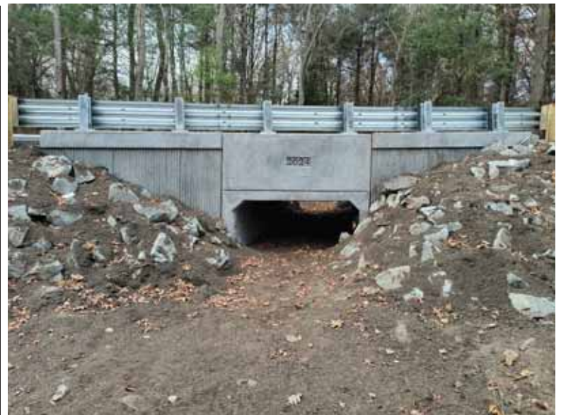
The newly upgraded Glendale Culvert (Photo: Ross Povenmire, Boxford Land Use Director)
